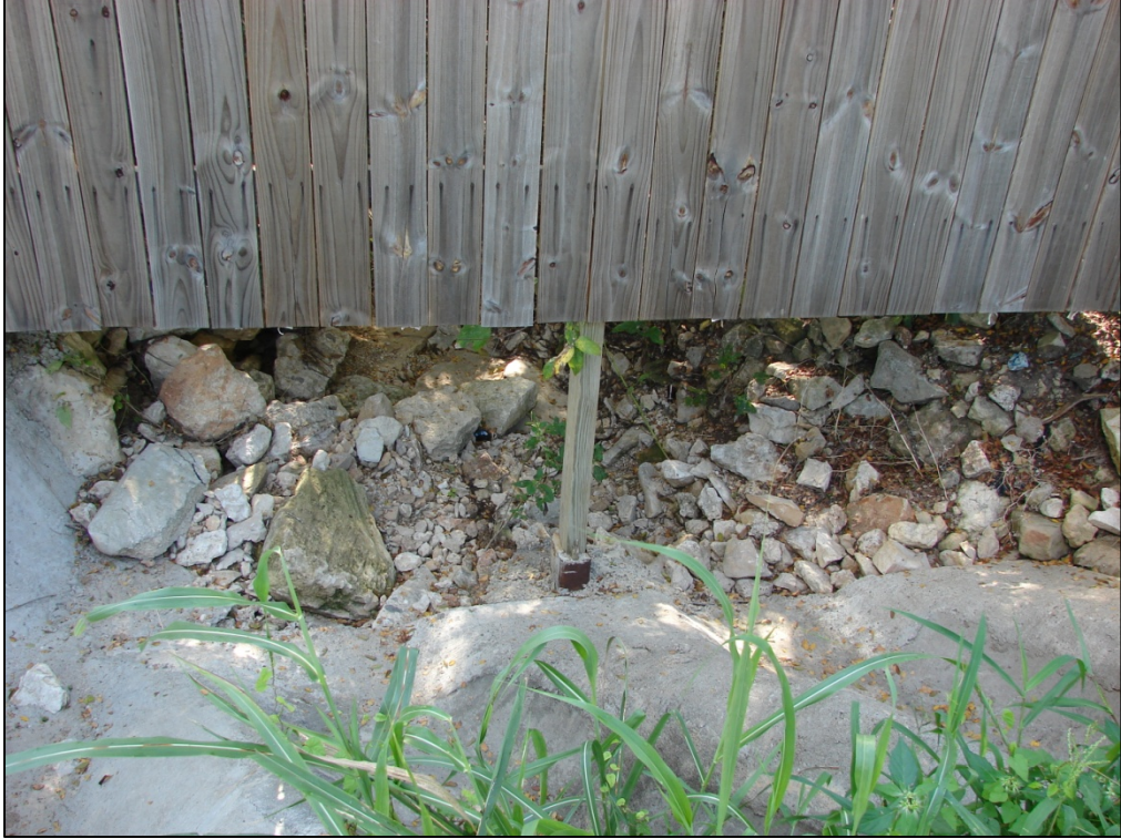
Photo 7: Entrance to drainage way east of North Meadowlark Street, facing southeast taken 9-21-2012
